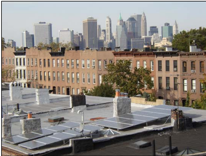
Figure 5.2: Photovoltaic System on a Rooftop in Brooklyn
